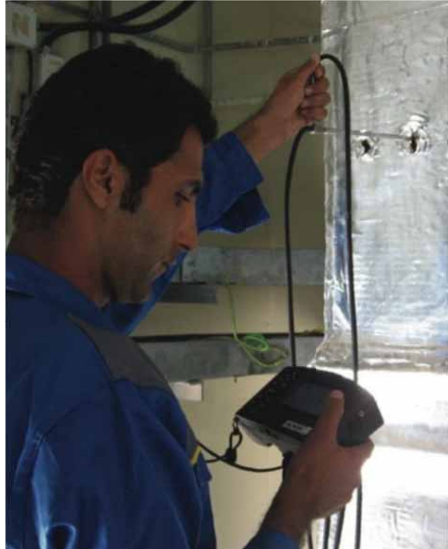
Performing combustion efficiency test
